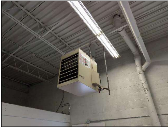
Photo 56. Typical open flame unit heater.
