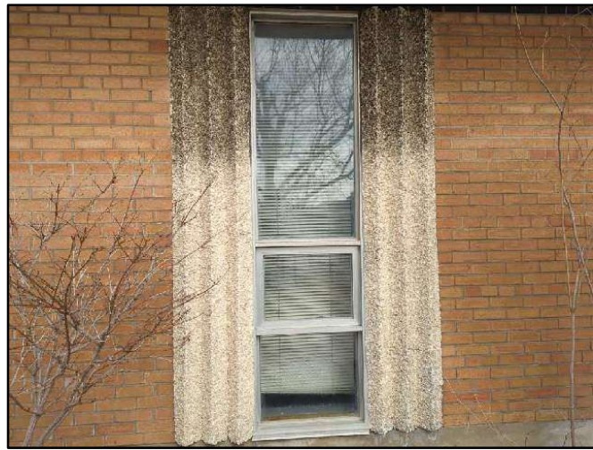
Photo 11. Example of a window with a lost seal. Note the condensation between the glazing.
