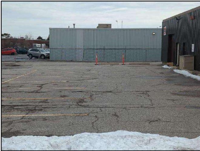
Photo 22. Example of cracking in asphalt paving at the north side of the property.
