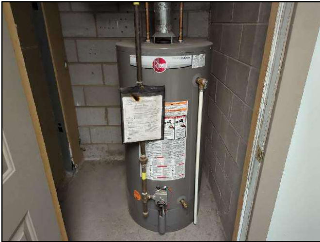
Photo 53. Gas-fired domestic water heater.
