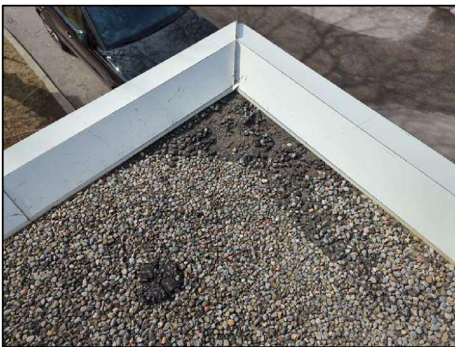
Photo 29. Wind scouring of gravel, exposing the membrane at the southwest corner of the lower level roof.
