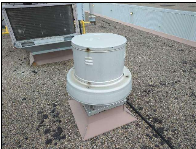
Photo 57. Typical rooftop exhaust fan for the office washrooms.
