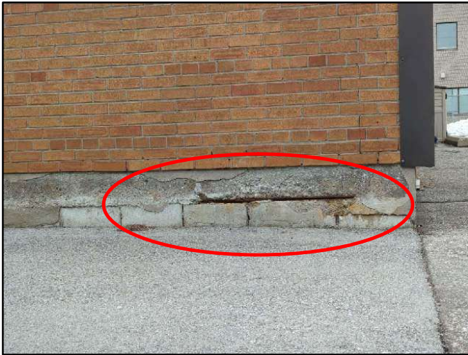
Photo 1. Deteriorated parging, localized spalling of the floor slab edge and exposed horizontal reinforcement at the northeast corner of the building.
