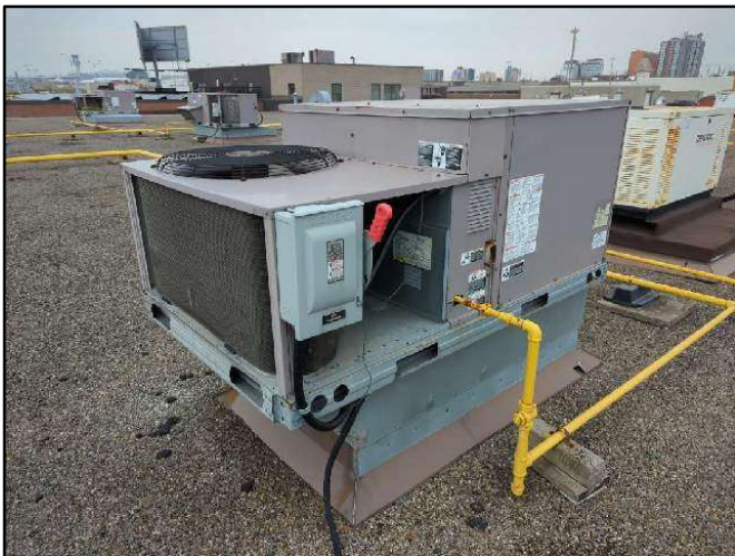
Photo 55. Typical rooftop heating and cooling unit.
