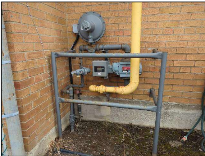
Photo 54. Gas meter for building.
