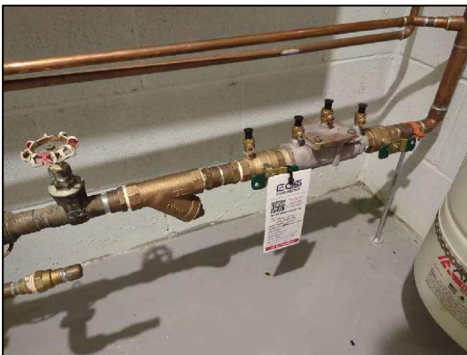
Photo 52. Backflow prevention device at the domestic water service entrance.
