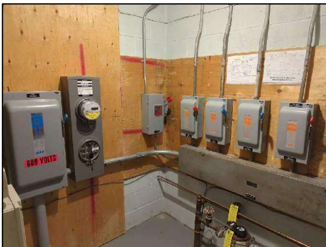
Photo 58. Overview of main electrical service entrance equipment.
