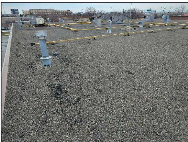
Photo 24. Overview of the built-up asphalt and gravel membrane on the upper roof level.
