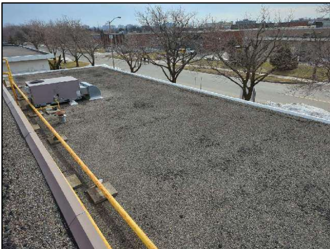
Photo 27. Overview of the built-up asphalt and gravel membrane on the lower level roof.
