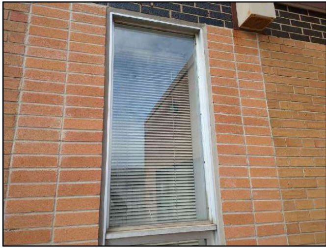
Photo 10. Example of a cracked window.
