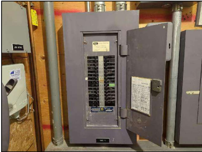
Photo 59. Typical circuit breaker panel.
