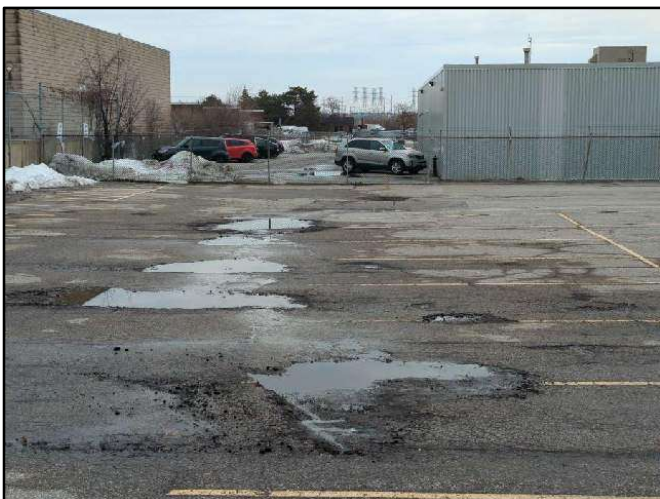
Photo 21. Example of potholes in asphalt paving at the north side of the property.
