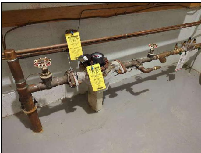
Photo 51. Main domestic water service entrance.
